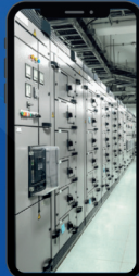
ELECTRIC PANEL BOARDS
